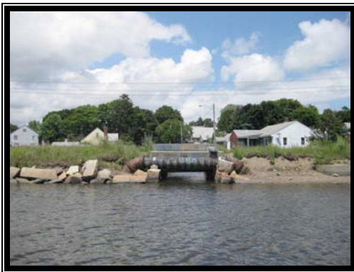
Old rail trail culverts at high tide on 09 July 2009. View looks north.
