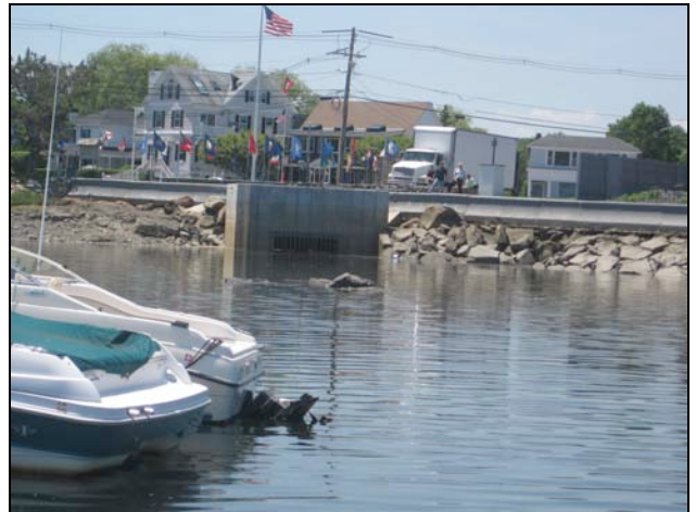
Tide gate located on Border Street. (TG)
